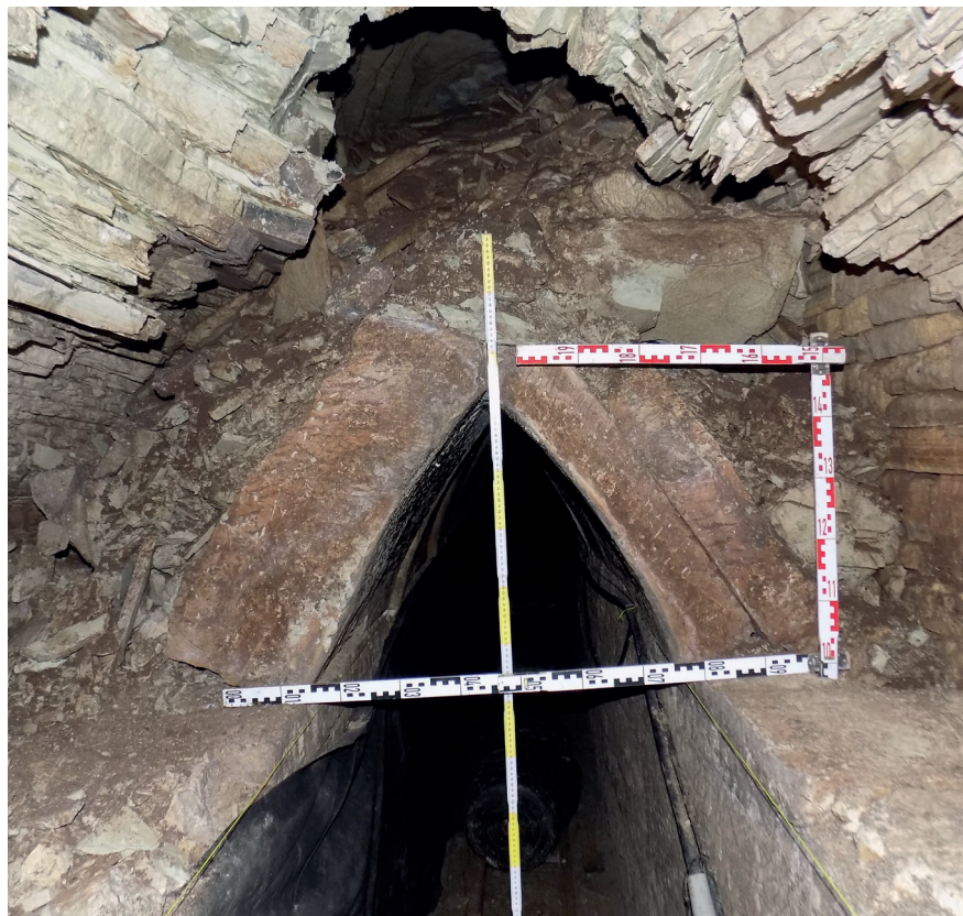
Fig. 22. The dismantling of the slabs of the archaic lining at Ch. 178.6, view from south
