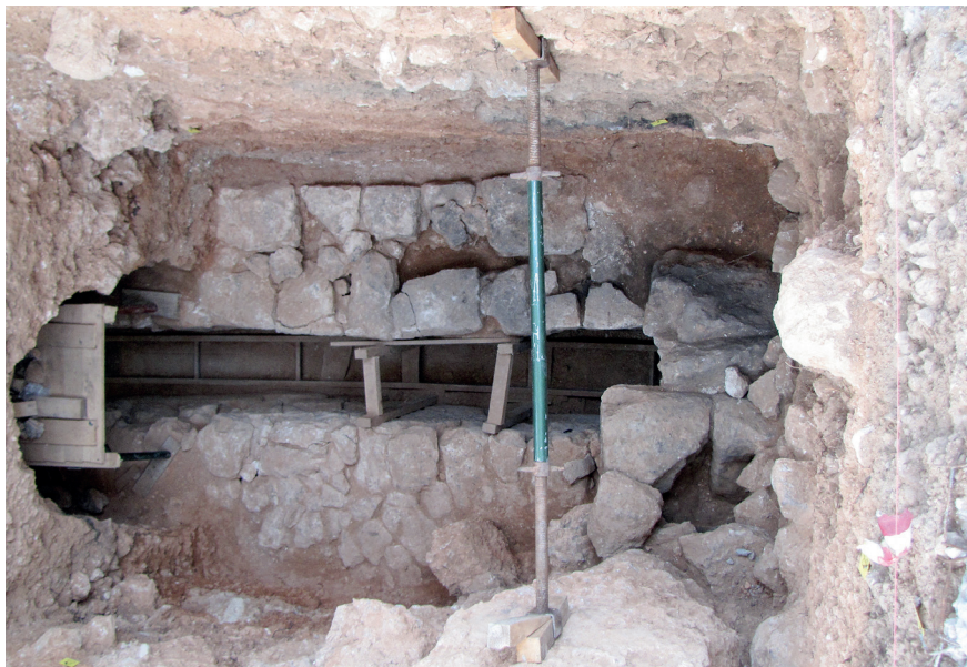
Fig. 23. The excavation near the south portal and the dismantling of the blocks of the roof of the Archaic lining, north on the left
