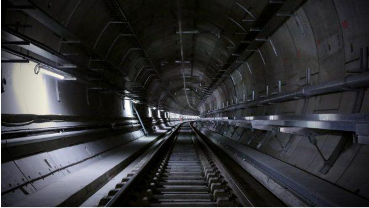
Overhead catenary system installed in Thames Tunnel_271050 DHLE installed in Thames Tunnel
