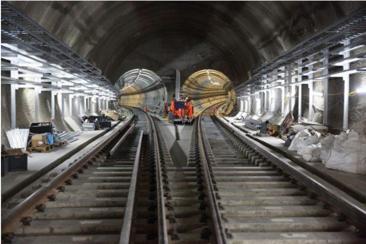
○ Cable management systems installed in Stepney Green eastbound cavern_270034
