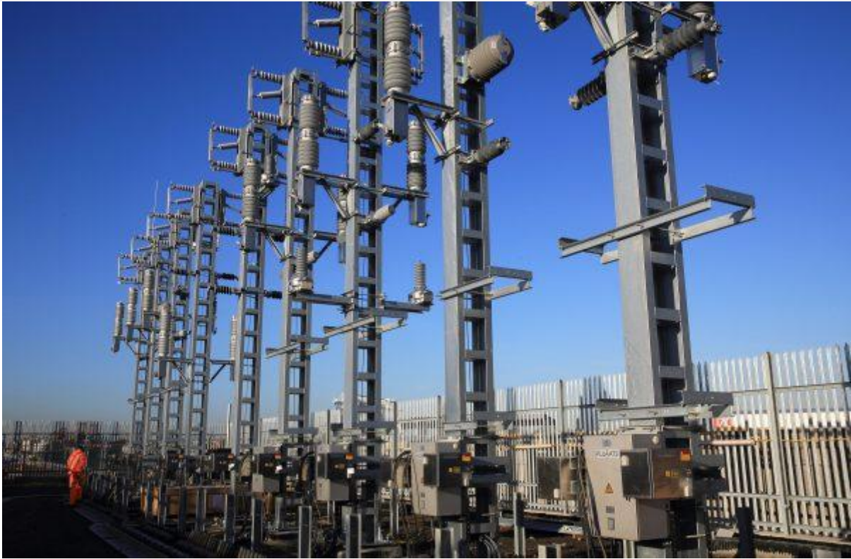
High voltage switchgear installed at Plumstead_257608
