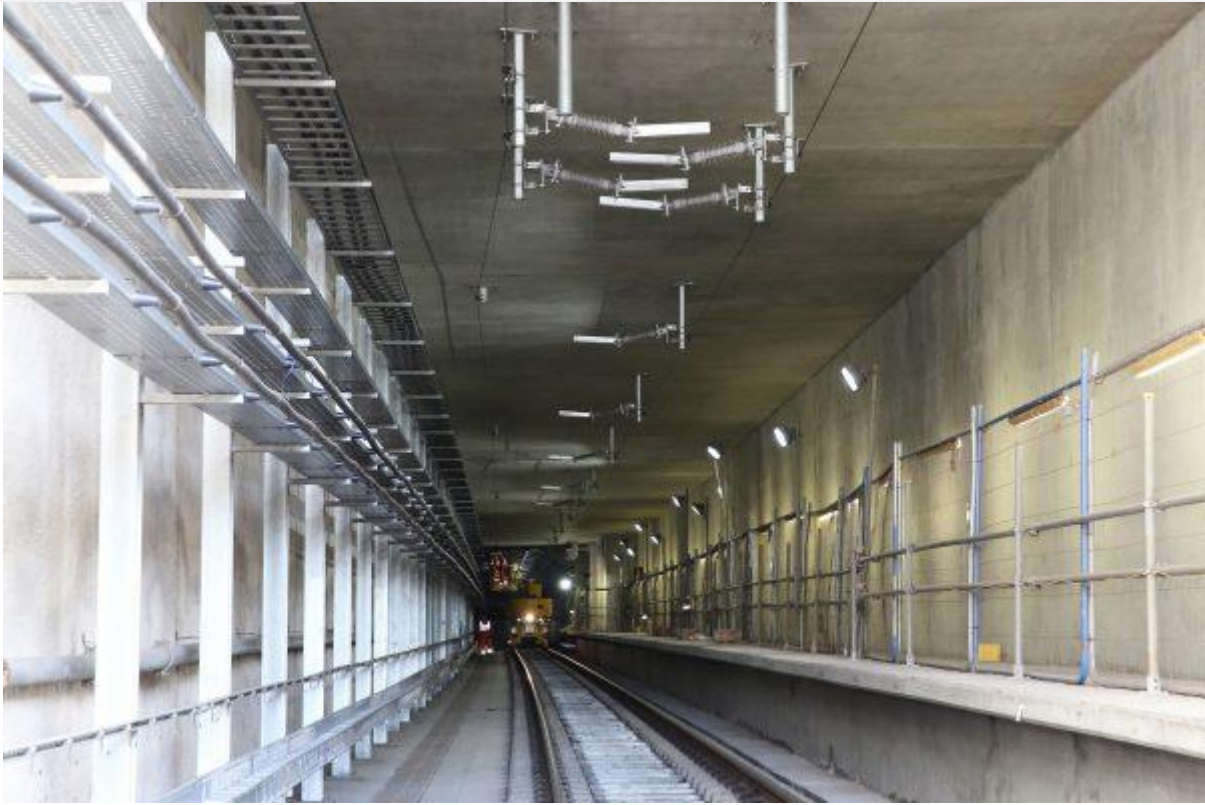
Overhead catenary system brackets and cable trays installed in entrance to Thames Tunnel_266095
