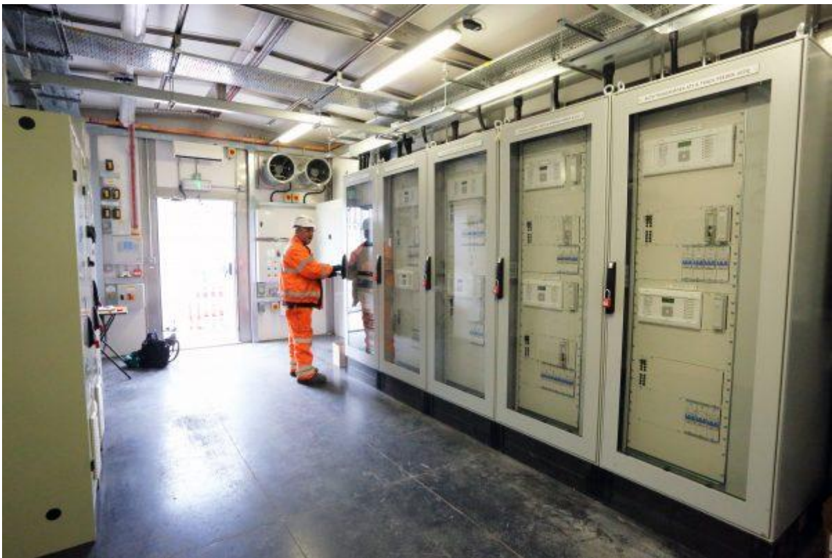
Control room being inspected prior to commissioning_270000
