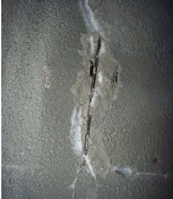
Figure 11a: Spalling of the shotcrete surrounding a highly stressed lattice girder.
