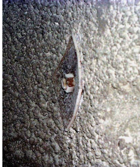
Figure 11b: Deformed rockbolt face plate due to overstressing of the primary support system.
