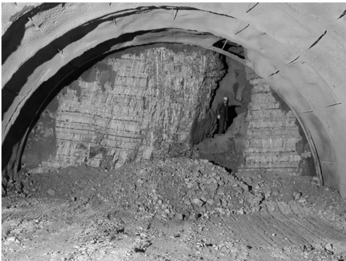
Figure 7: Typical appearance of a small karstic void partially filled with clay and silt; Dodoni Tunnel, northwest Greece, 2000 (Photo taken from site engineer)
