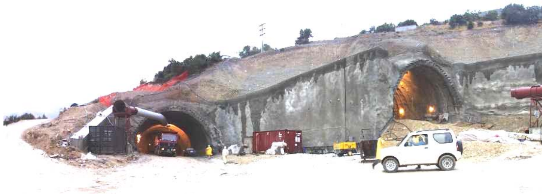
Figure 19: Current appearance of the portals for Tunnel S3 in Section 5.2.3. Note the very shallow cover over the tunnels.
