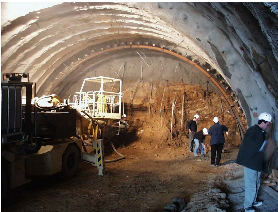
Figure 18: Appearance of face of tunnel S4 under construction. Depth below surface 40 m and maximum recorded displacement is 45 mm. Support: 12 m long 114 mm diameter forepoles at 0.6 m centres, steel sets with elephant foot support, fibre-reinforced shotcrete and fibreglass face reinforcement
