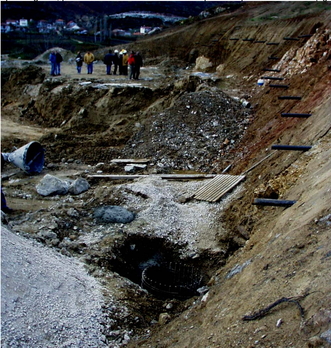
Figure 16: West portal excavation for S4 tunnel. Drainage pipes are shown projecting from the slope and a partially completed cast in place pile is shown in the foreground.
